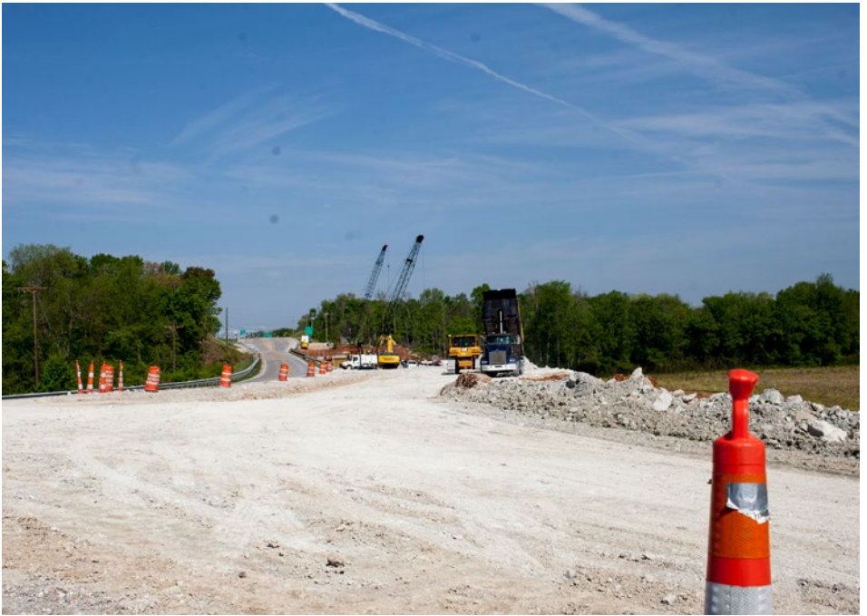
Construction crews work on the bridge over Drakes Creek on Cemetery Road (KY 234).
