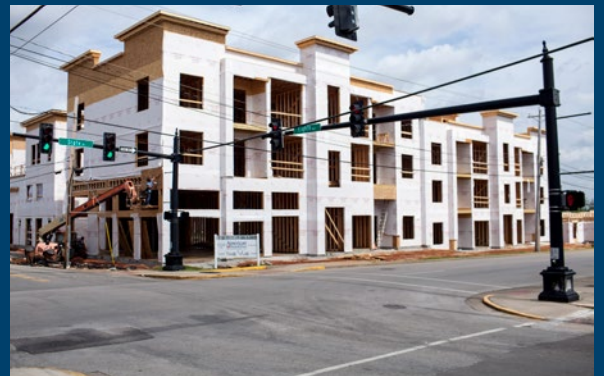
Construction of mixed-use development in Downtown Bowling Green, one of the many changes reflecting growth in the MPO area.
