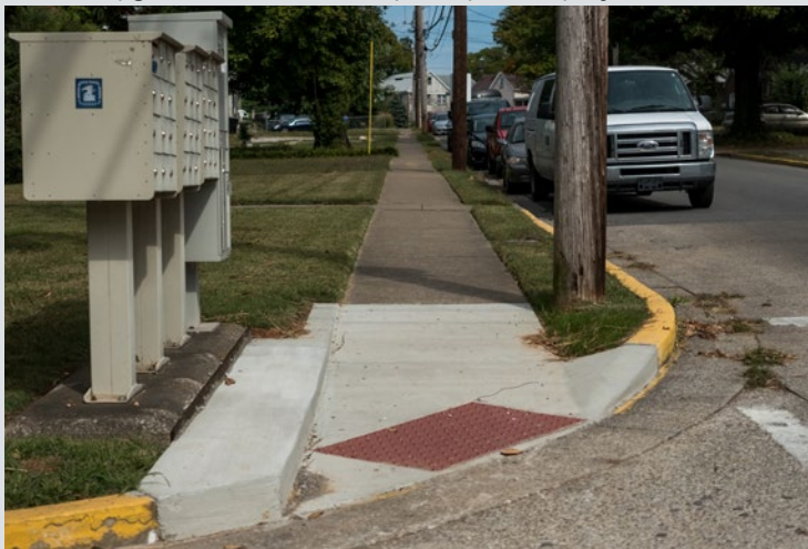
Curb ramp repairs to meet ADA compliancy on Cabell Drive, at the intersection with Ogden Avenue/High Street.
