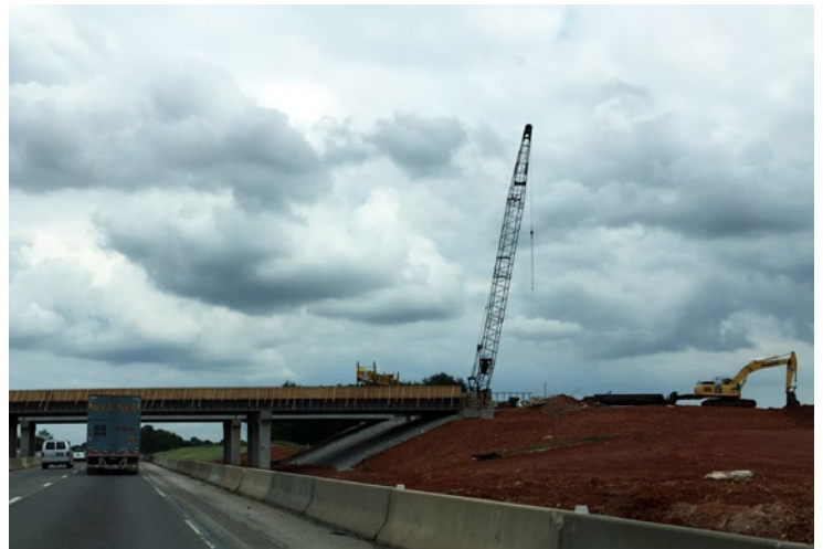
I-65 to U.S. 31W connector project, traveling north on I-65 near exit 28.
