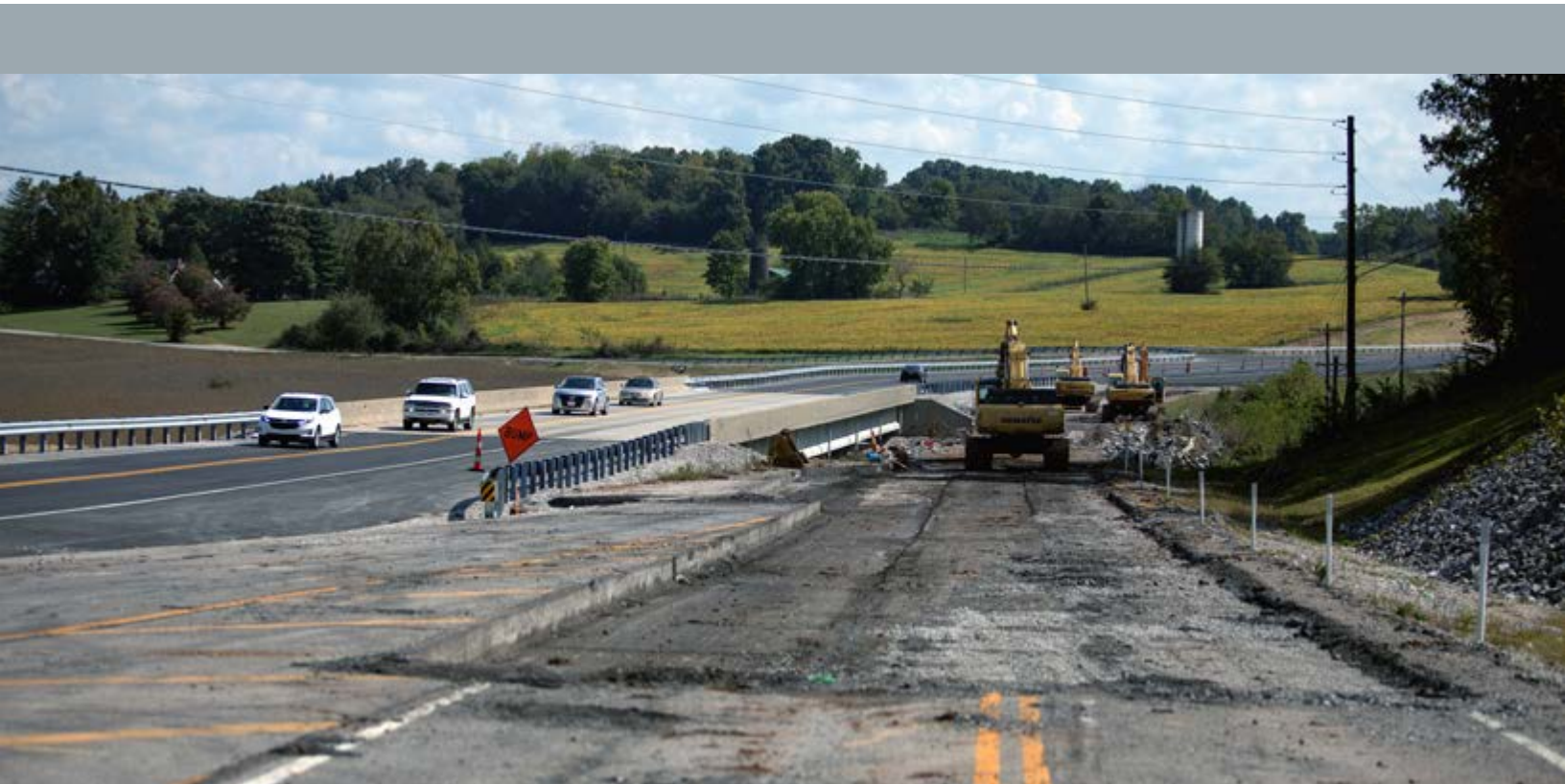
Construction crews work on the KY 234 (Cemetery Road) bridge over Drakes Creek.
