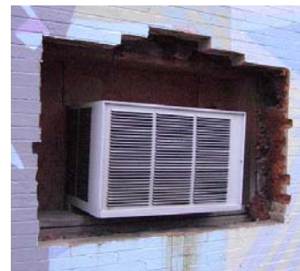
It is not appropriate to cut an historic masonry wall for a heating or cooling unit or even a new window.
