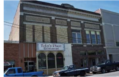
Backlit signs are not appropriate for a property with Local Historic Designation. New owners have replaced this inappropriate sign with a sign on their awning.
