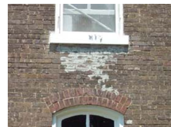
Before the Rose-Daughtry house came under the care of Warren County Parks it was inappropriately patched with concrete.
