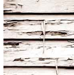
Extensively deteriorated paint needs to be removed to bare wood, then primed and re-painted. Photo: NPS files.
