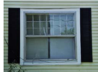
This is an example of inappropriate shutters since they clearly would not cover the entire window, if they were closed and, in addition, are made of a synthetic material.
