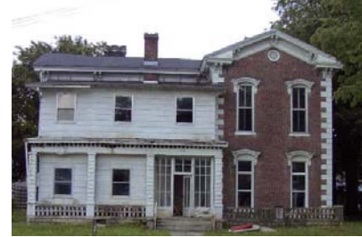
The porch of this home was enclosed to create additional living space but in doing so completely destroyed the personality of the house. A rear addition would have been more appropriate. Since this photograph was taken, new owners have constructed a historically appropriate porch.
