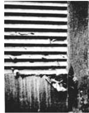
Here, a latex top coat was applied directly over old oil paint, resulting in intercoat peeling. The latex was unable to adhere. If latex is used over oil, an oil-base primer should be applied first. Photo: Mary L. Oehrlein, AIA.
