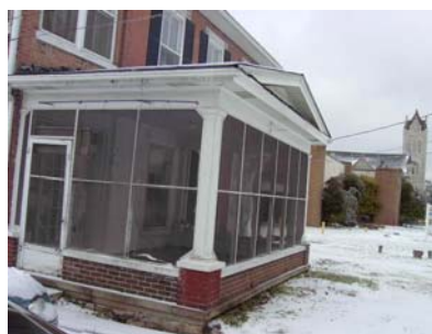
This front porch on State Street has been enclosed with wood framed screens—an appropriate method for enclosing a front porch.
