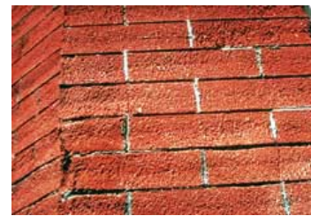
Sandblasting has permanently damaged this brick wall. Photo: NPS files
