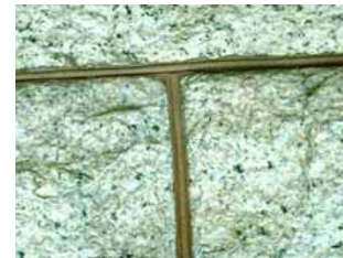
This late 19th century granite has recently been repointed with the joint profile and mortar color carefully matched to the original. Photo: NPS files.
