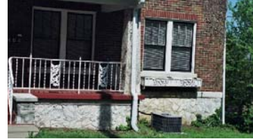
A more appropriate location for the HVAC unit below this front window would have been the rear or the side of the house.
