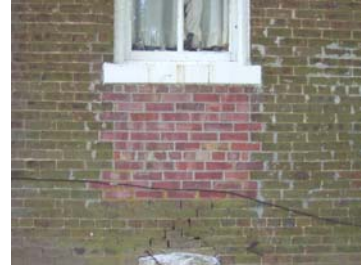
The brick on this house was inappropriately patched. The current owners might choose to repair the patch with more appropriate mortar and brick or they may choose to paint the house.
