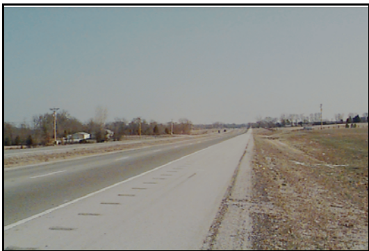
U.S. 68-KY 80, a major arterial traversing Warren County from the southwest to the northeast, was upgraded in the early 1990's.
